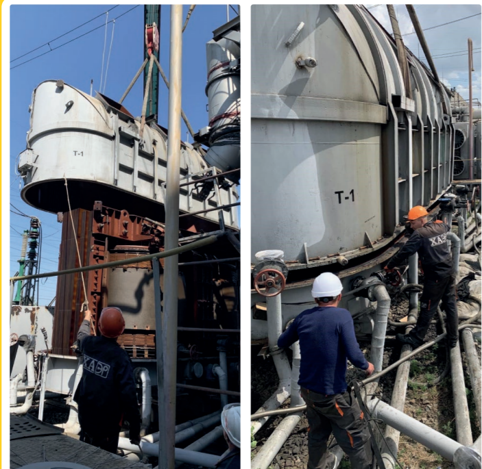
Repair work for the ТДЦГ-400000/154 unit transformer and the boiler gas ducts at Unit 1 at Kryvyi Rih CHP, DTEK Dniproenergo.
