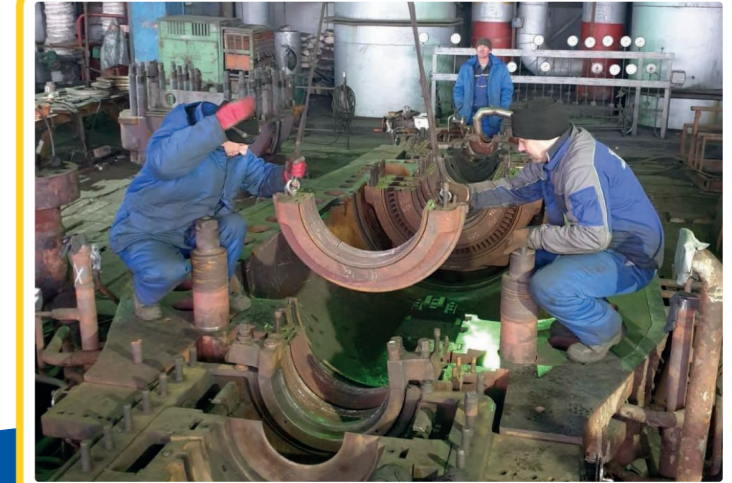
Major overhaul work for the K-300-240 turbine at Trypilska TPP, Centrenergo PJSC, which was carried out during and after air strikes in the winter time in the turbine hall with shattered windows.
