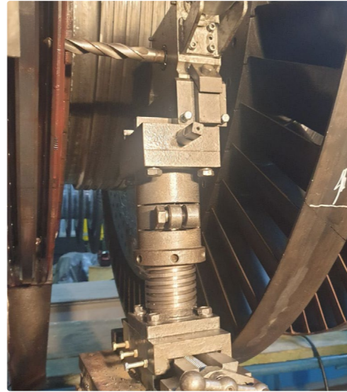
Major overhaul work for the K-200-130 turbine, Unit 5, at Zmiivska TPP, Centrenergo PJSC, which was shut down several times after repeated missile strikes during repair work.
