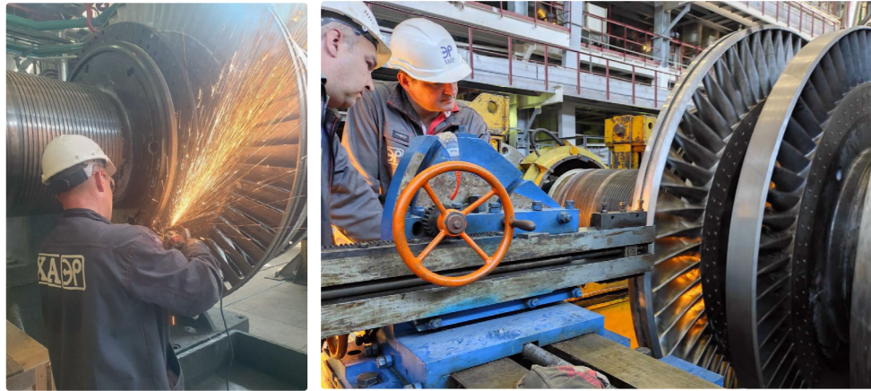
Emergency repair work for the high-pressure rotor of the 1000 MW K-1000/3000 turbine, Unit 2, at Khmelnytskyi NPP, National Nuclear Energy Generating Company Energoatom.
