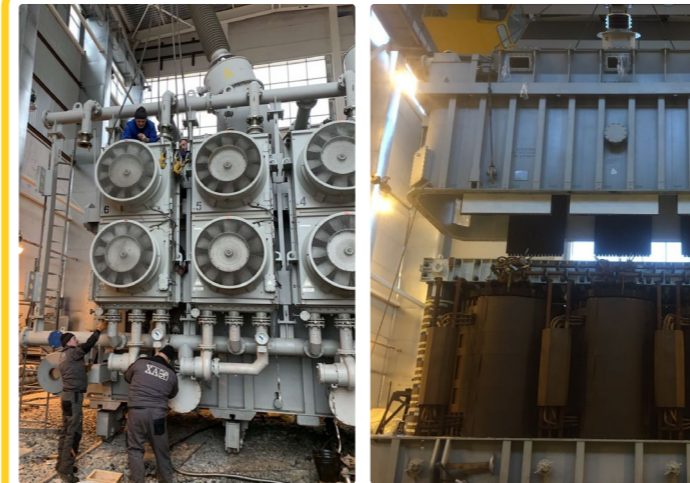
Repair work for the Т4 ТДЦ-430000/330-У1 transformer at Dniester PSPP, Ukrhydroenergo PrJSC, to identify the source of gas release.
